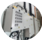
Panel Shops & Control Boards
